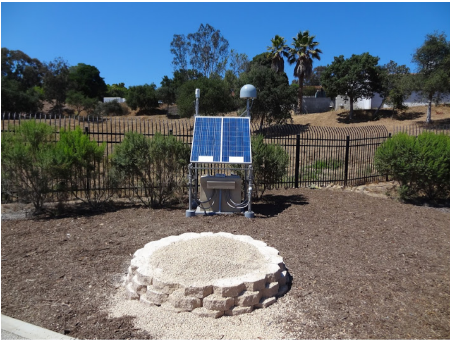
Figure 2. Station EOCG at the Santa Barbara Emergency Operations Center. Seismic vault is located in the foreground. Photo courtesy of Dan Determan, USGS. Photo was taken sometime between July and December 2014.
